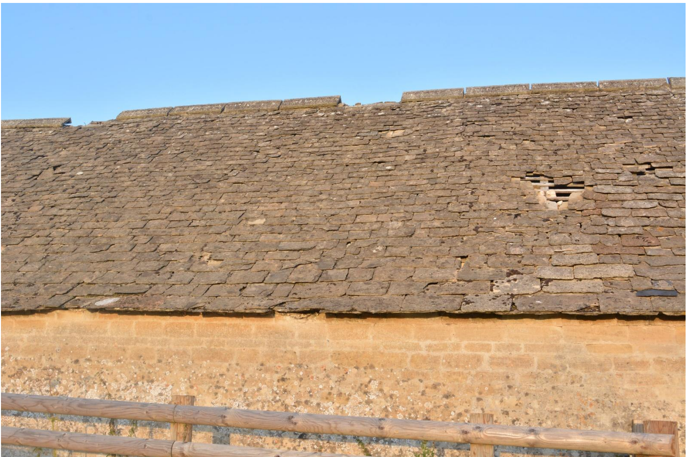
Western elevation roof deterioration: as above and missing ridge tiles.
