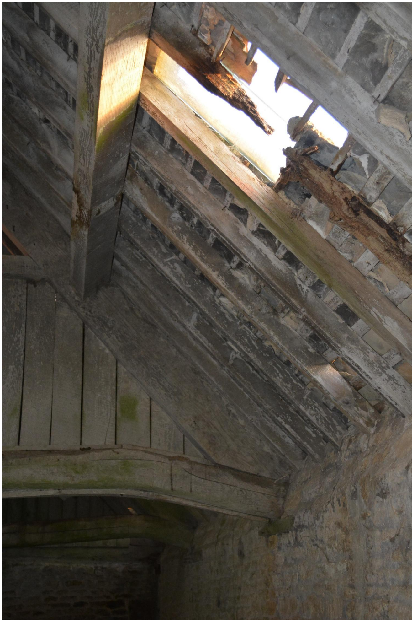
Interior detail: west facing roof of western barn showing rotten rafters and open void. Note original roof Trusses with curving tie beams.
