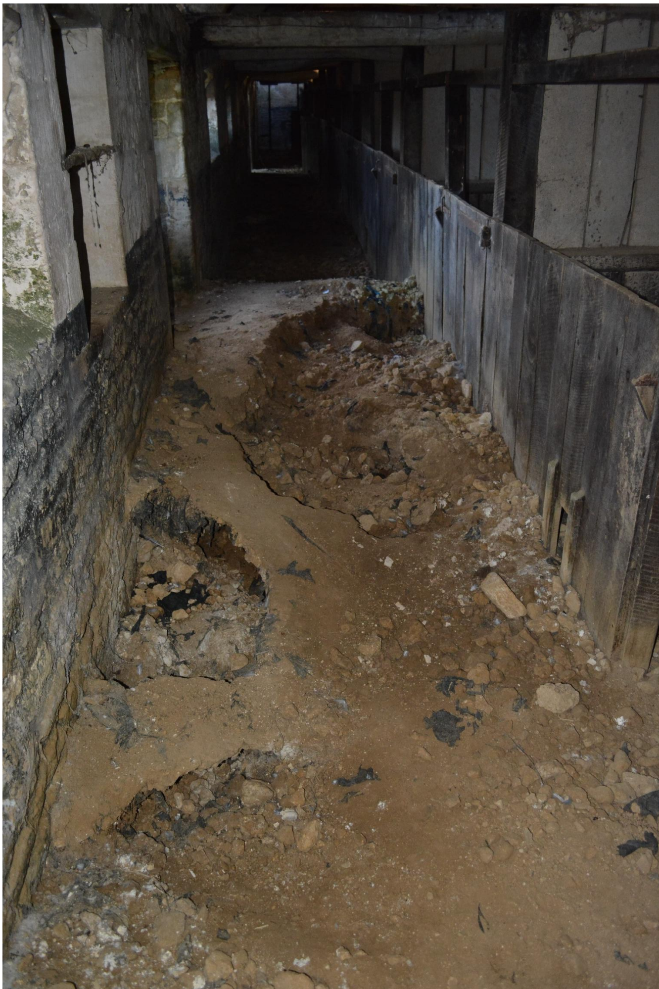
Interior detail within the northern barn showing active badger sett and excavations within the floor. Note the original timber stalls to the right.
