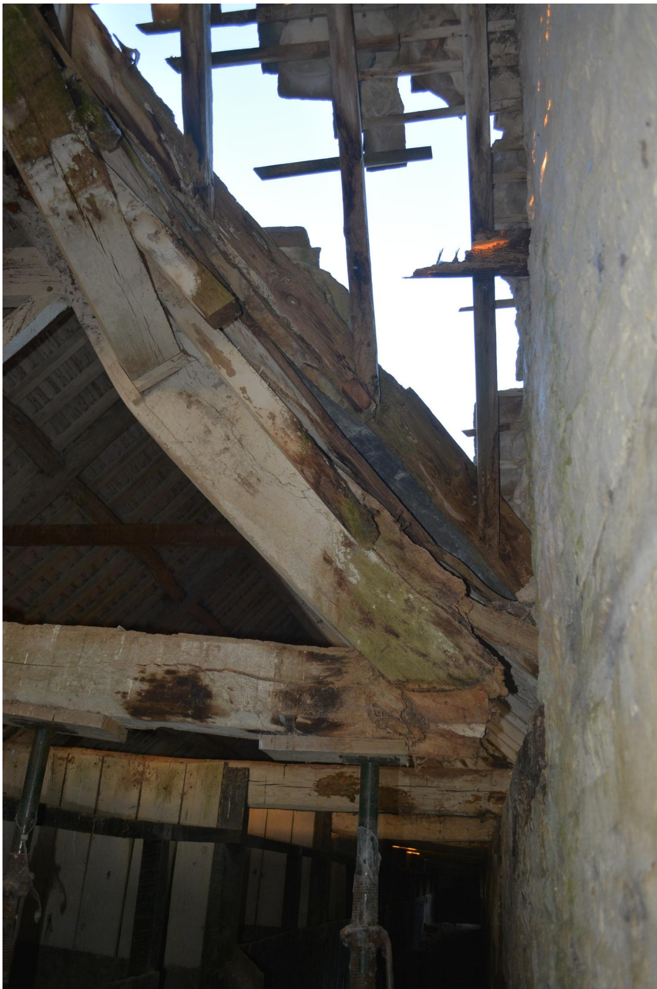
Interior detail: south facing roof of northern barn showing rotten and collapsed roof truss and open void.
