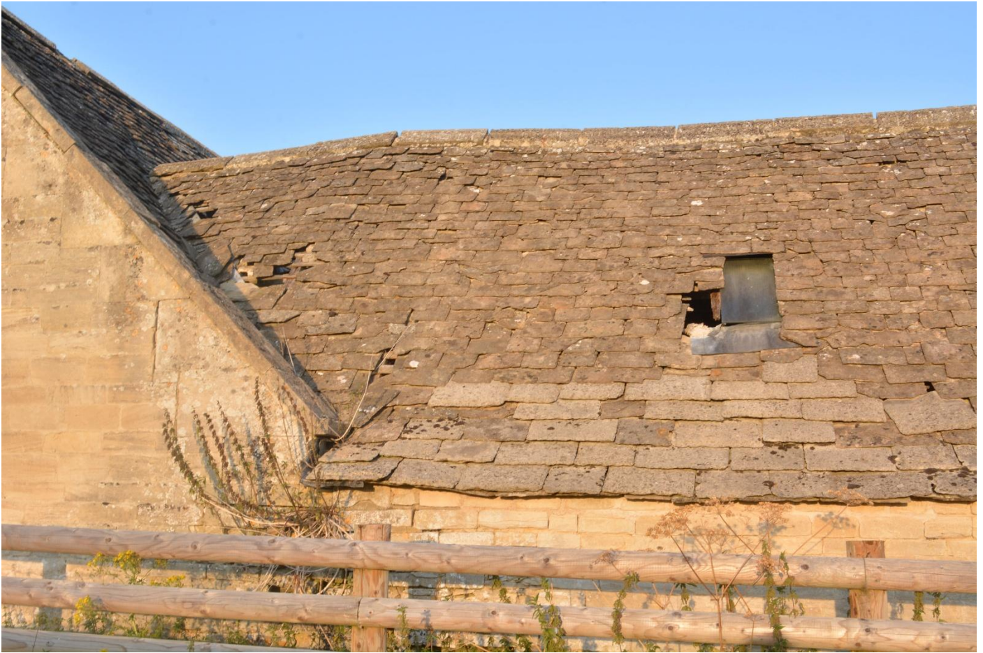
Western elevation roof deterioration: missing slates, open voids, collapsed ridge, replacement concrete slates.
