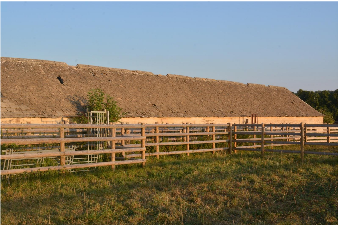
Western elevation. Note holes in the roof, missing / slipped slates and missing ridge tiles.
