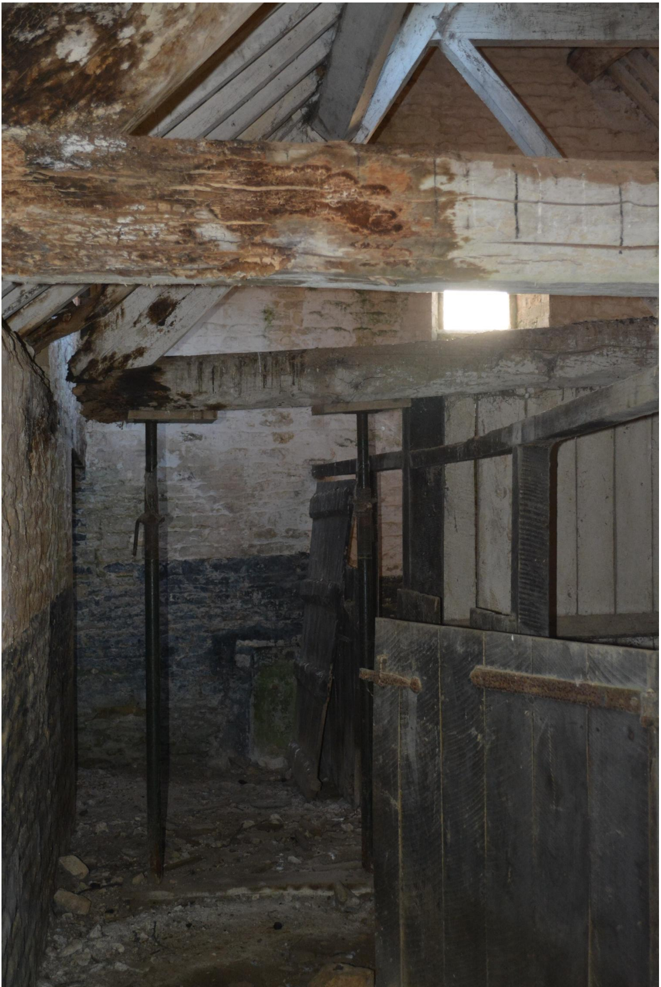
Interior detail: western end of northern barn showing collapsed roof truss.
