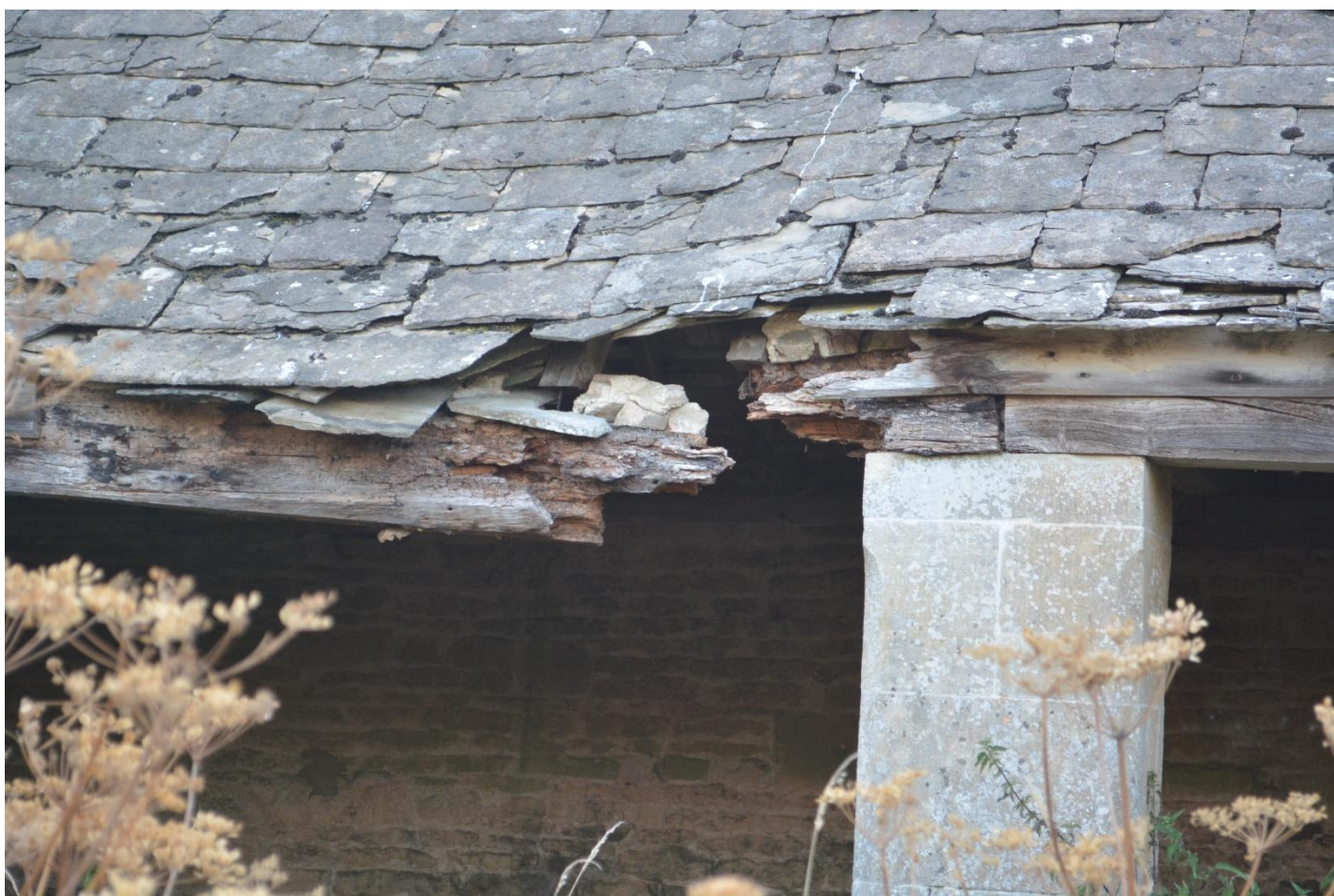
East facing elevation on interior courtyard showing rotten and collapsed timber lintel between stone piers.
